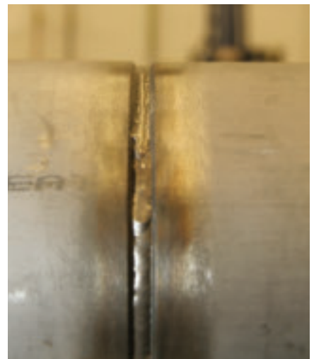
A root bead that is too convex can lead to fusion problems.
