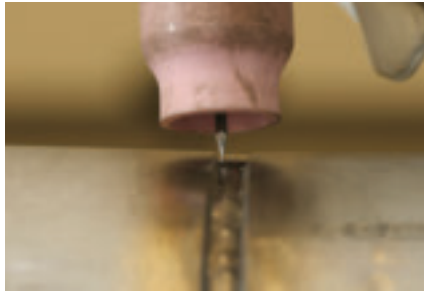
When welding a pass freehand, pause at the side of the weld to allow the pool behind the arc to solidify.
